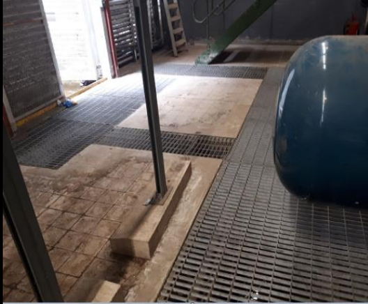
Figure 1: Evidence of Slips, Trips and Falls Finding
