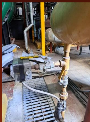
Figure 4: Evidence of manual gas isolation valve
